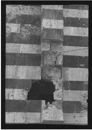
SC-016_13985_066.tif Damaged monuments P
