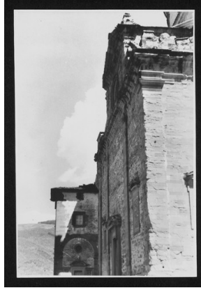
SC-016_13977_063.tif Damaged monuments C
