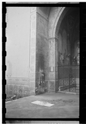
SC-016_13985_108.tif Damaged monuments P
