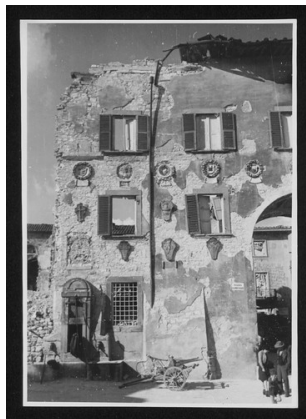
SC-016_13985_043.tif Damaged monuments P
