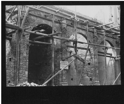
SC-016_13979_017.tif Damaged monuments E
