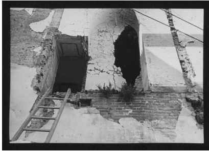
SC-016_13985_075.tif Damaged monuments P
