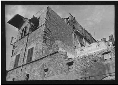
SC-016_13985_069.tif Damaged monuments P
