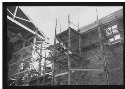
SC-016_13985_082.tif Damaged monuments P
