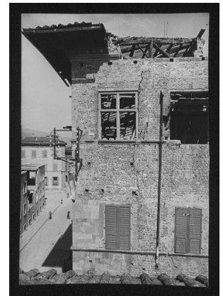
SC-016_13985_071.tif Damaged monuments P
