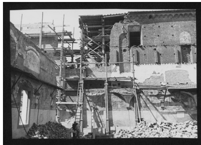
SC-016_13985_073.tif Damaged monuments P
