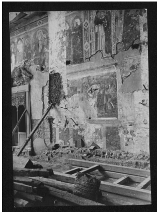
SC-016_13985_078.tif Damaged monuments P
