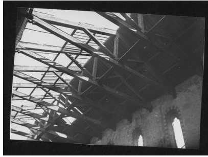
SC-016_13985_067.tif Damaged monuments P
