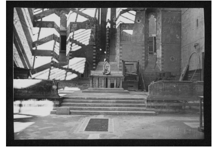
SC-016_13985_068.tif Damaged monuments P
