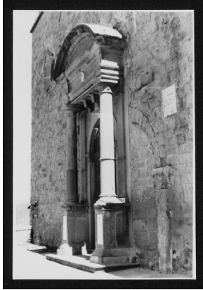
SC-016_13977_062.tif Damaged monuments C
