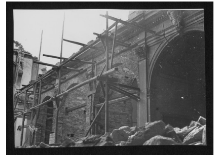
SC-016_13979_019.tif Damaged monuments E
