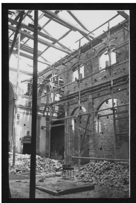
SC-016_13979_020.tif Damaged monuments E
