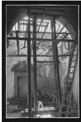
SC-016_13976_018.tif Damaged monuments B
