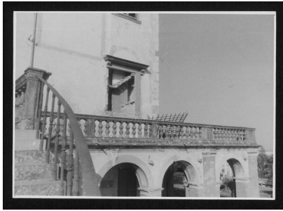
SC-016_13985_003.tif Damaged monuments P
