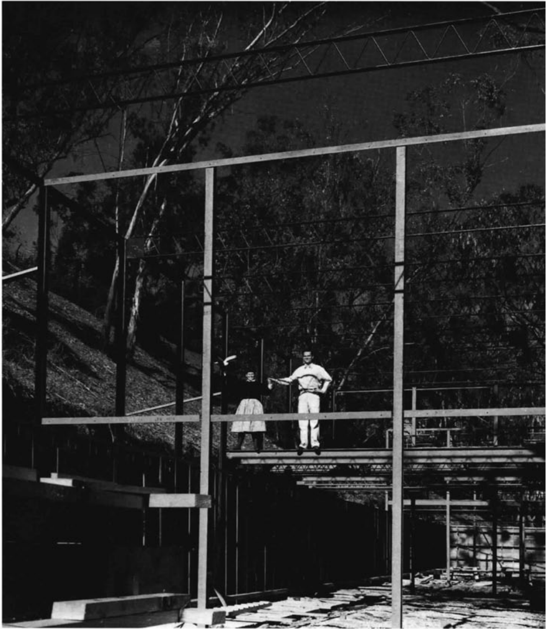
Charles (right) and Ray Eames on the steel frame of the Eames House, Pacific Palisades, California, 1949. Photograph: John Entenza
