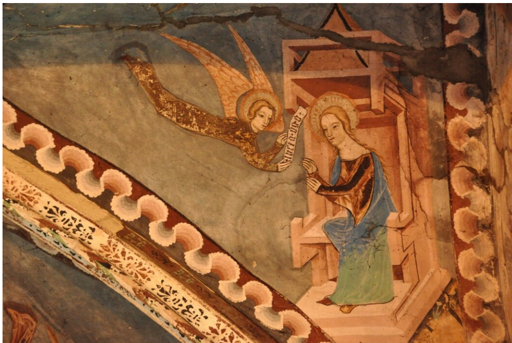
Fig. 10. Wall painting in the Church of the Virgin Mary, Mălâncrav, Transylvania, Romania. Detail. Note the color change of the Virgin Mary's mantle from blue to green due to formation of hydroxy copper chlorides.
